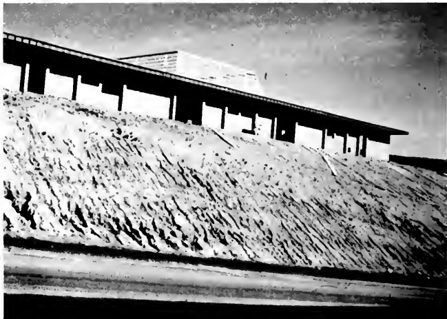
Photo 20. Rills from rainwash visible, but no cracks developed in fill materials or structures. Engineered fill placed under modern techniques and caides.
